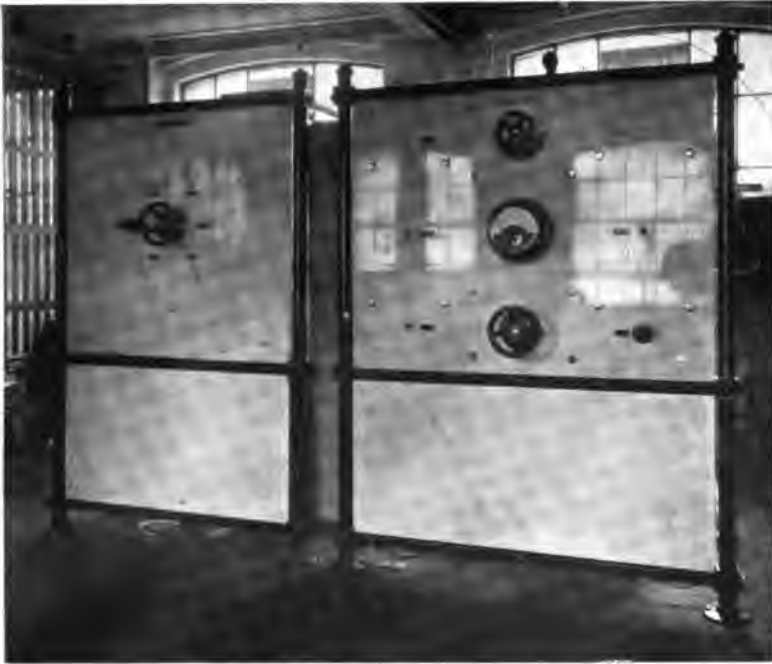
FIG. 141.—Front of excitation and aerial lengthening coil panels (15 T.K.). Siemens Bros. & Co., Woolwich.
